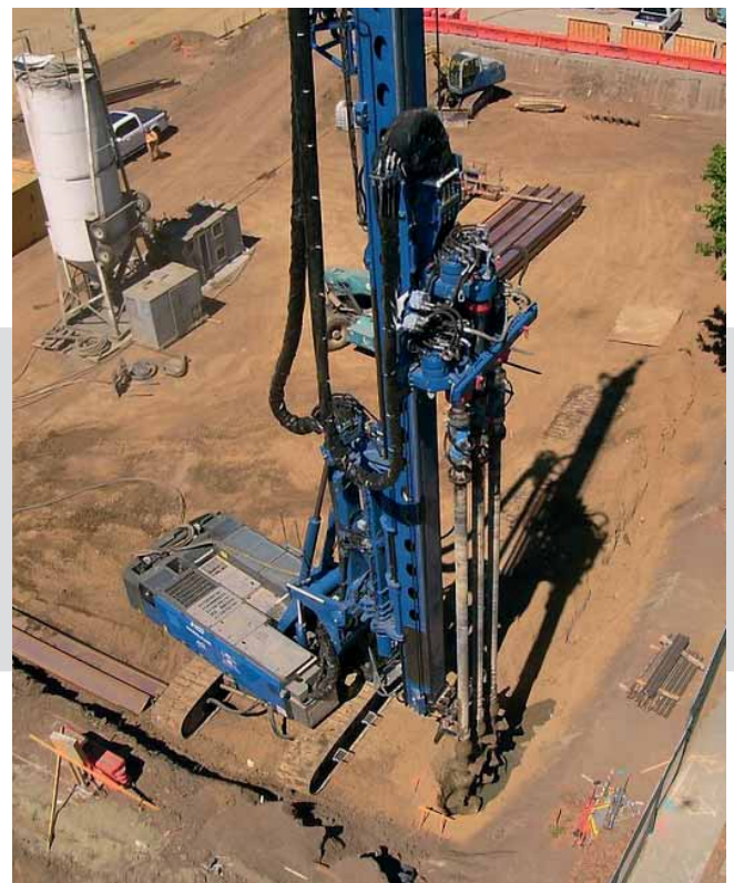
Soil mixing with the Triplemix auger drive. In one step three overlapped mixed piles are installed.
