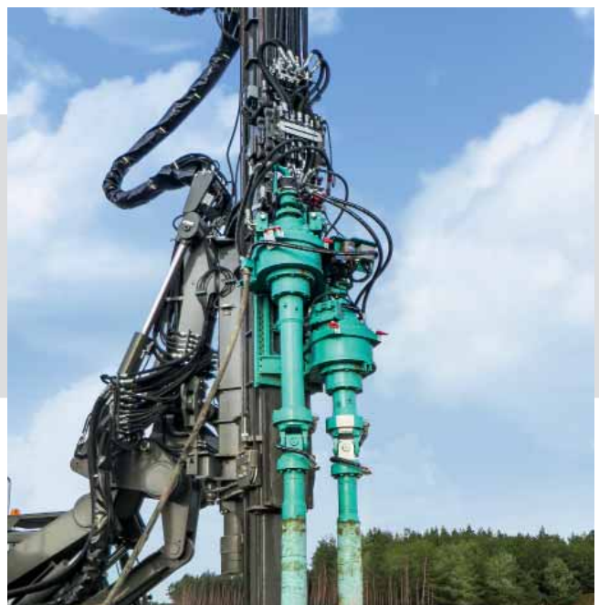
For soil mixing, productivity can be increased by using multiple auger drives.
