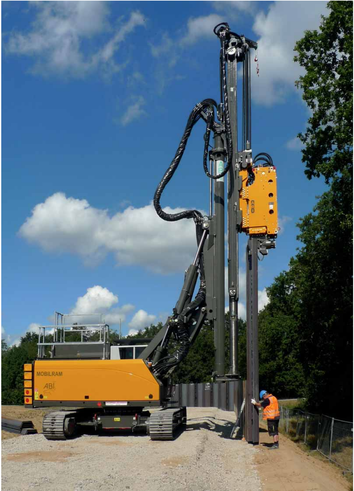
A classical application for the ABI MOBILRAM-System with vibrator: The installation of a sheet pile wall.
