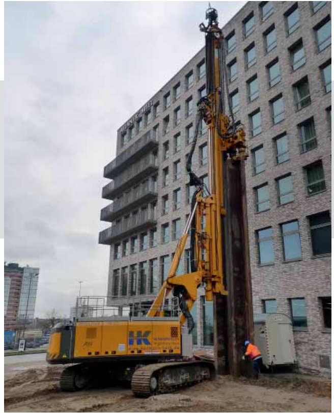
Static pressing directly in front of existing buildings. In some cases the soil must be loosened by pre-drilling before pressing.
