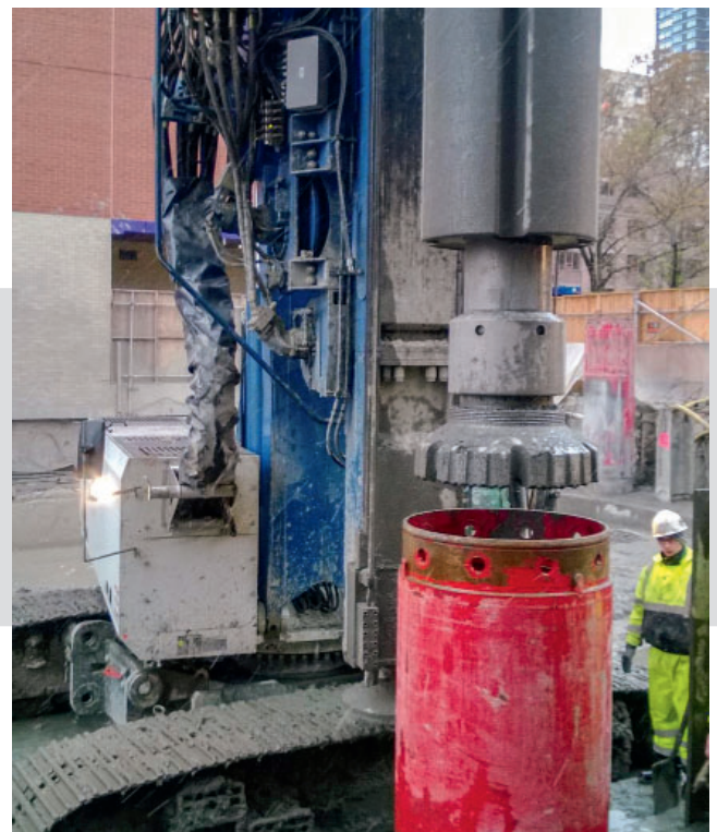
DELMAG drill rig using a down the hole hammer in hard, rocky ground.
