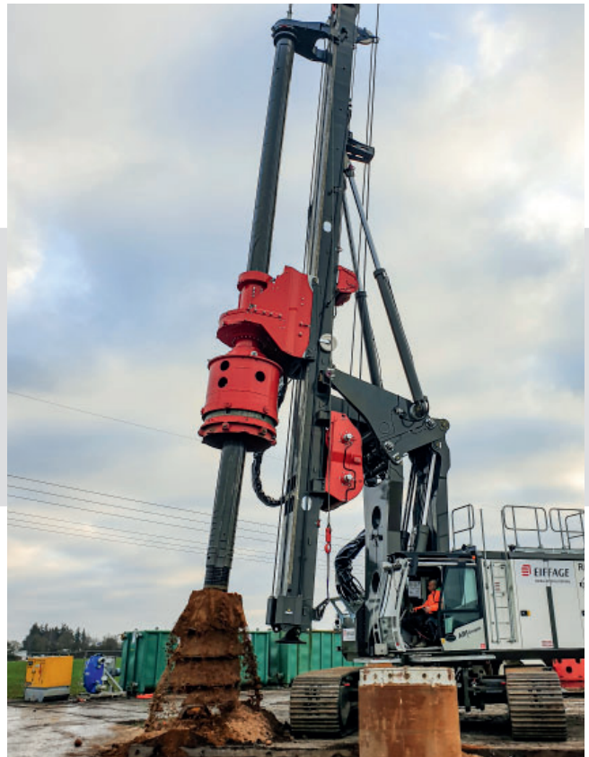
Drill rig with Kelly bar guide: In the case of inclined piles, the Kelly bar is also guided at the upper end to prevent the Kelly bar from tipping.
